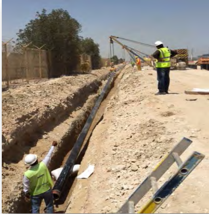
CCS Facility Mussafah Section
