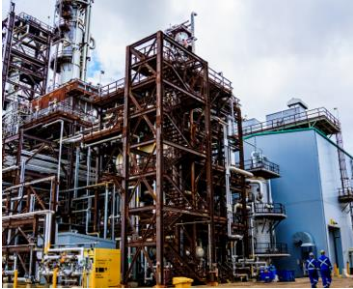
CO 2 capture at the NWR Sturgeon Refinery
