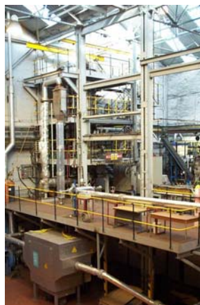
Doosan Babcock Emissions Reduction Test Facility
