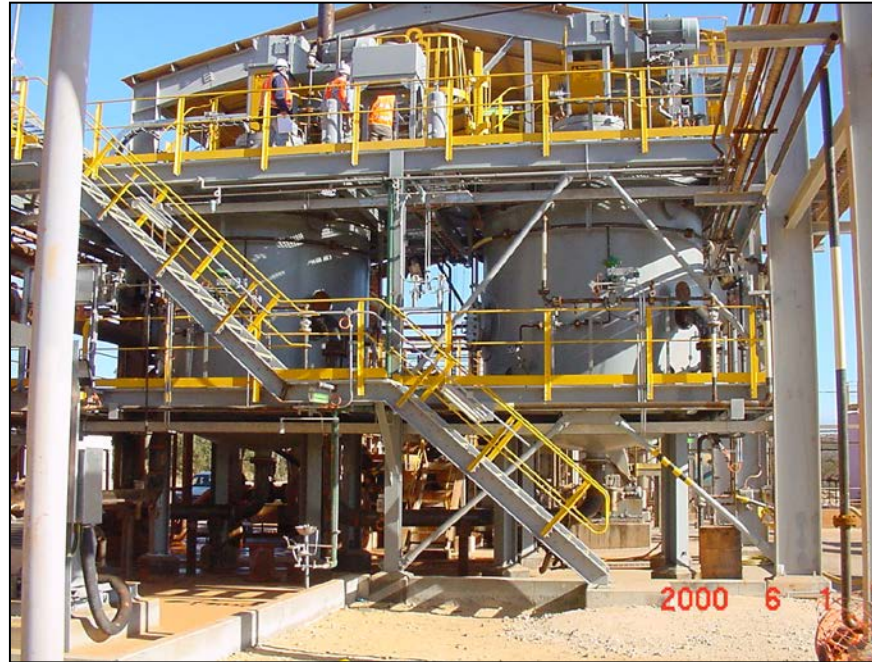
CO 2 mixing tanks
