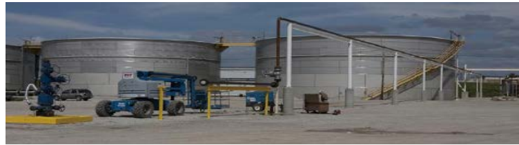
CO 2 Pipe to Injection Well
